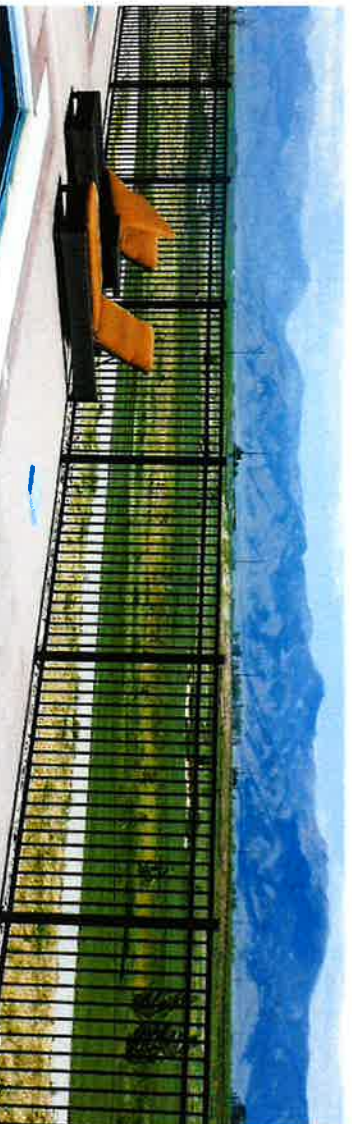
Tubular Steel Fence & Pilasters - 4' height
