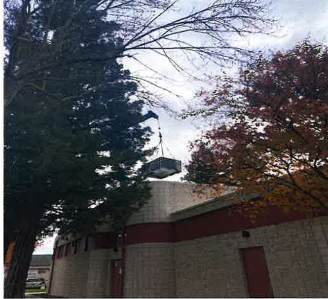
New HVAC unit at Community Center
